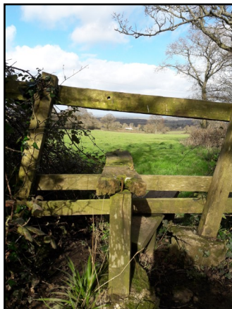
Stile in need of repair
